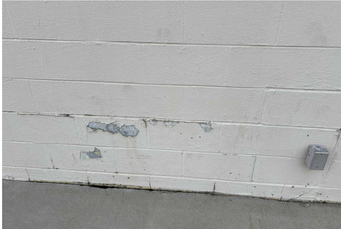
North inside wall; paint bubbling; repainted almost annually
